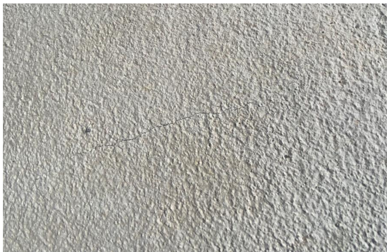
Plate 15: Typical Plastic Shrinkage Cracking - icubed consulting
