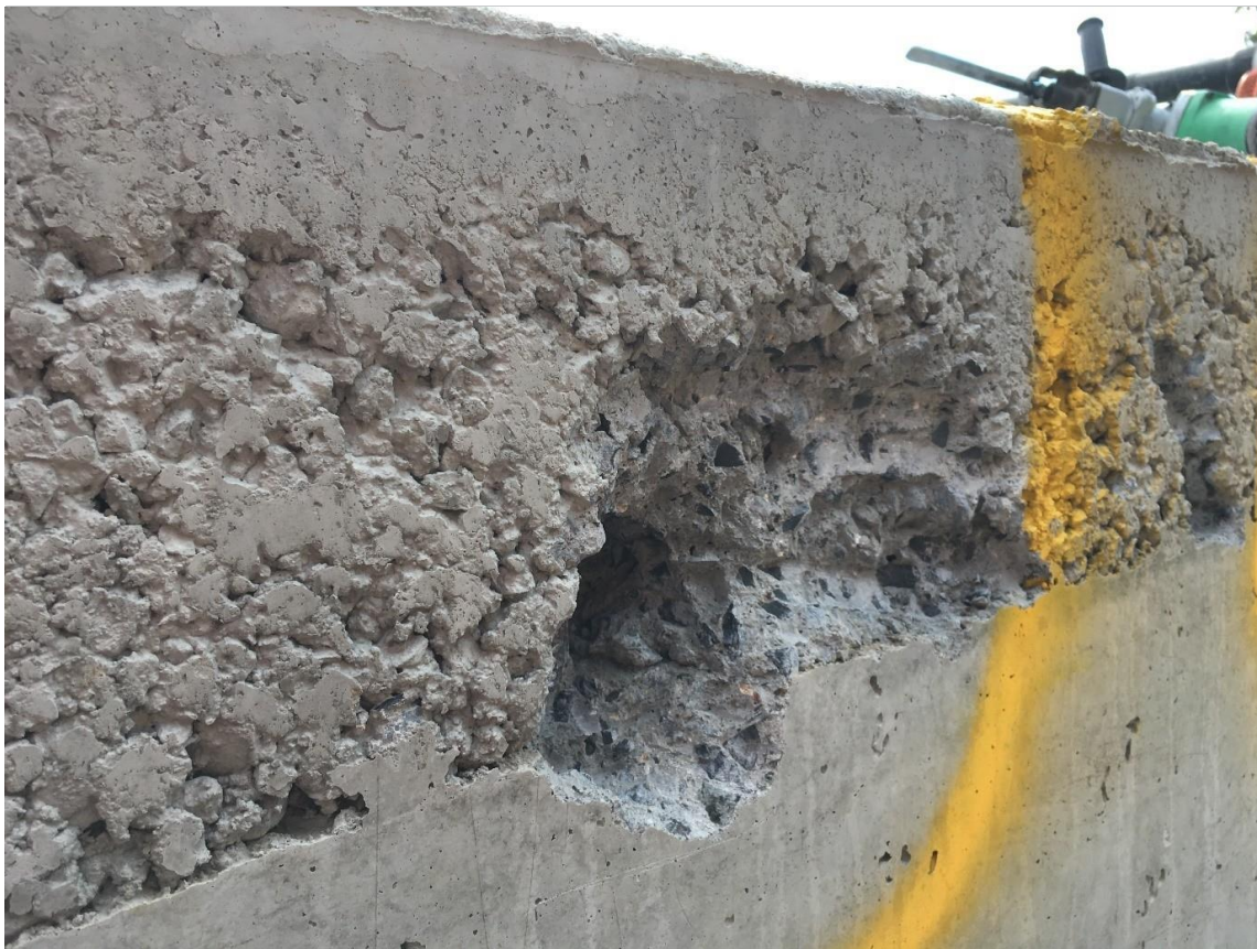
Plate 14: Example of cold jointing and under-vibration against the edge formwork - icubed consulting.
