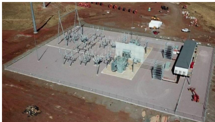
Plate 1: 220/33kV Substation – Dundonnell Windfarm, Victoria
