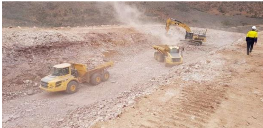
Plate 22: Deep Cutting Spoil used for Rock Fill and Processed for Pavement Materials - Lincoln Gap Wind Farm, South Australia
