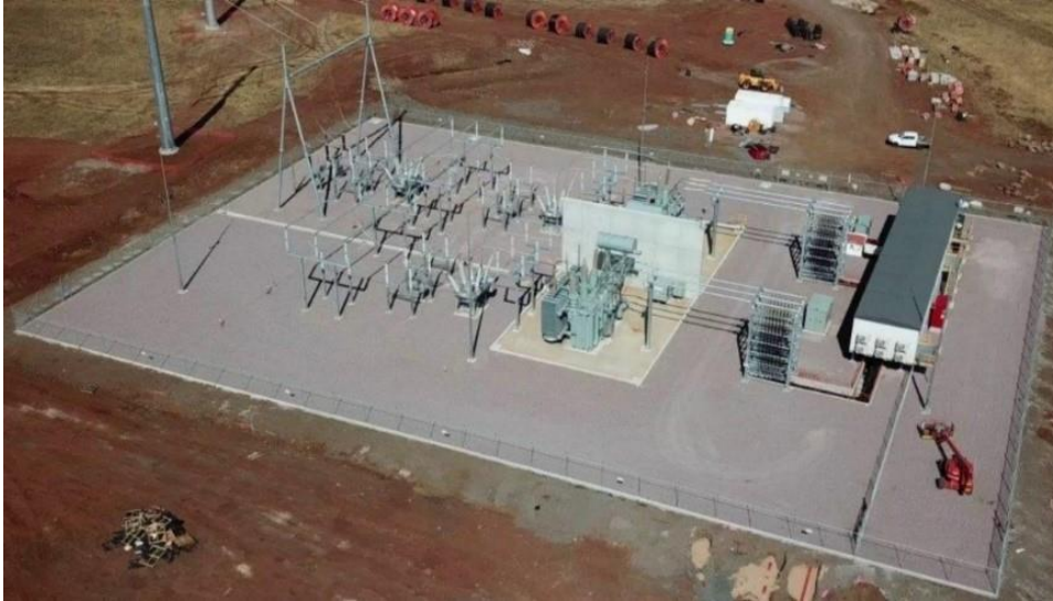
Plate 1: 220/33kV Substation – Dundonnell Windfarm, Victoria
